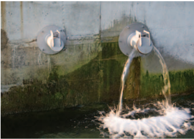
Figure 2: Water Outflow Point
